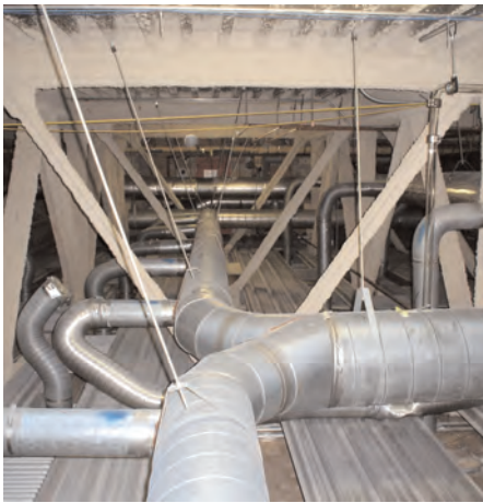
Asbestos fireproofing before Encasement
